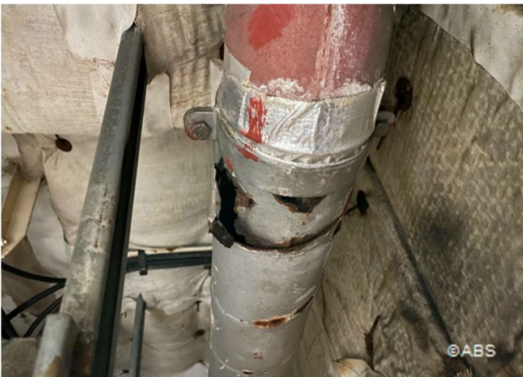
Holed ventilation ducting.
