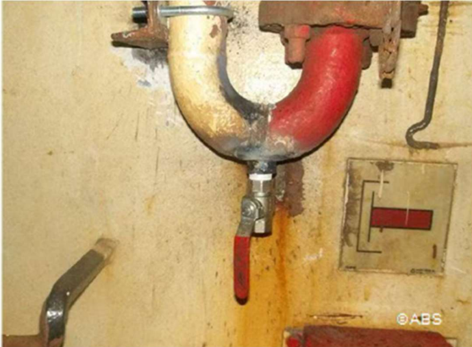
No drainage arrangement is provided at the bottom of the U-shape fire line on both sides of the main deck. Picture posted after rectification of finding.
