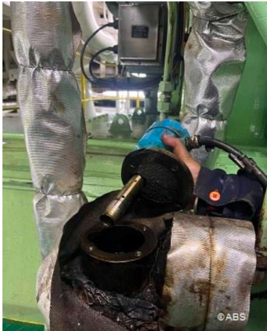
Top cover of Main Engine Fuel Oil leak-off alarm bypassed. Sensor was removed from alarm assembly.
