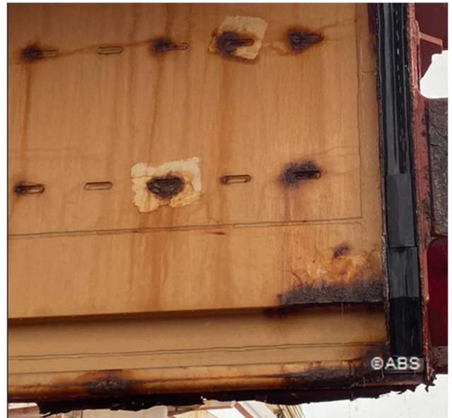
Hatch cover rubber packing found damaged or partially missing.
