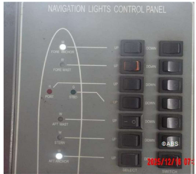
The aft mast light and forward anchor light are out of order.
