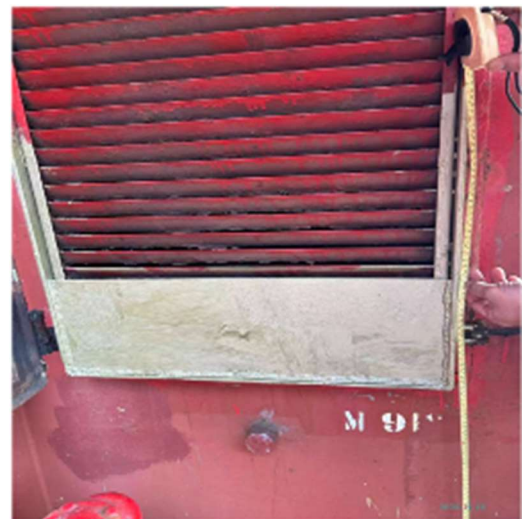
Height of the ventilators at poop deck was modified to 900mm. The original height during PSC inspection was 720mm. Per Load Line Convention/Regulation 19, ventilators in position 1 shall have a coaming height of at least 900mm.
